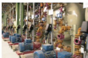
Picture 8: Pump room with plugs and sockets for up to 32 A (source: Bayer AG).
